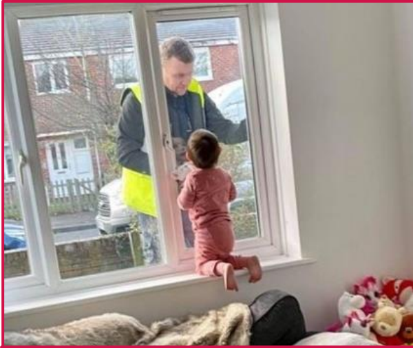
One of our repair men made a friend. While repairing a window, he the house's youngest resident entertained while he got the job done. Providing some smiles to our residents through a difficult time.
